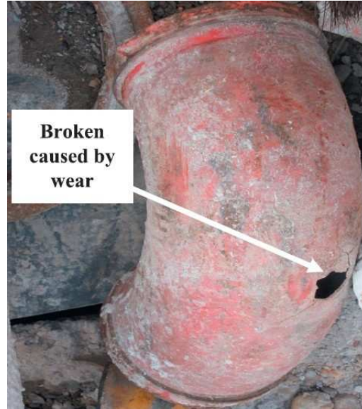
Figure 6.11: The destroyed pipe.
